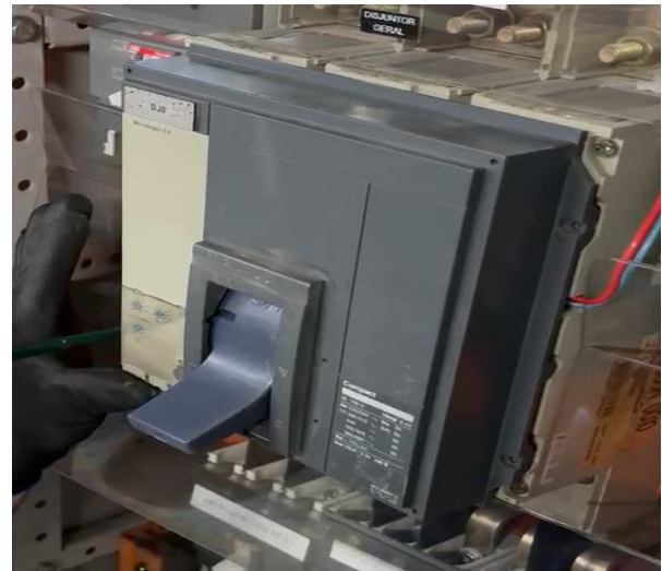
Figure 6. Manufactured part being used in the circuit breaker
