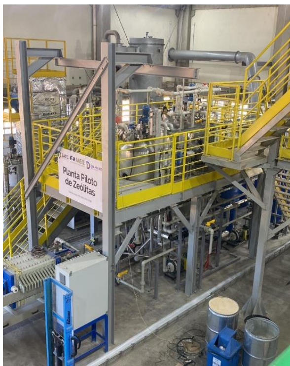
Fig.1. Zeolite Pilot Plant.
