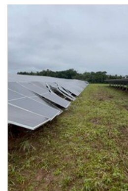
Figure 3. Panels after floods
