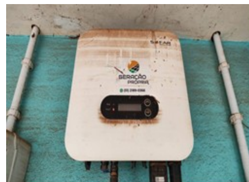
Figure 2. Inverter damaged by flooding
