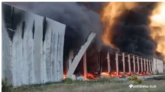
Fig. 5 Cladding panels strongly deformed and collapsed in the Taranto fire (2024)
